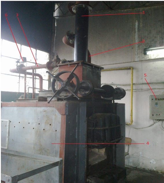
Figure 7. Fixed hearth furnace room 1. PAR-MD radiation preheater
