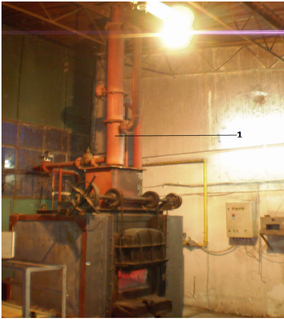
Figure 6. Fixed hearth furnace room 1. Preheater old radiation
