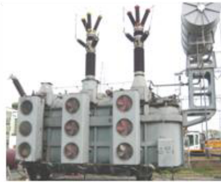
Figure 1. The power transformer.
